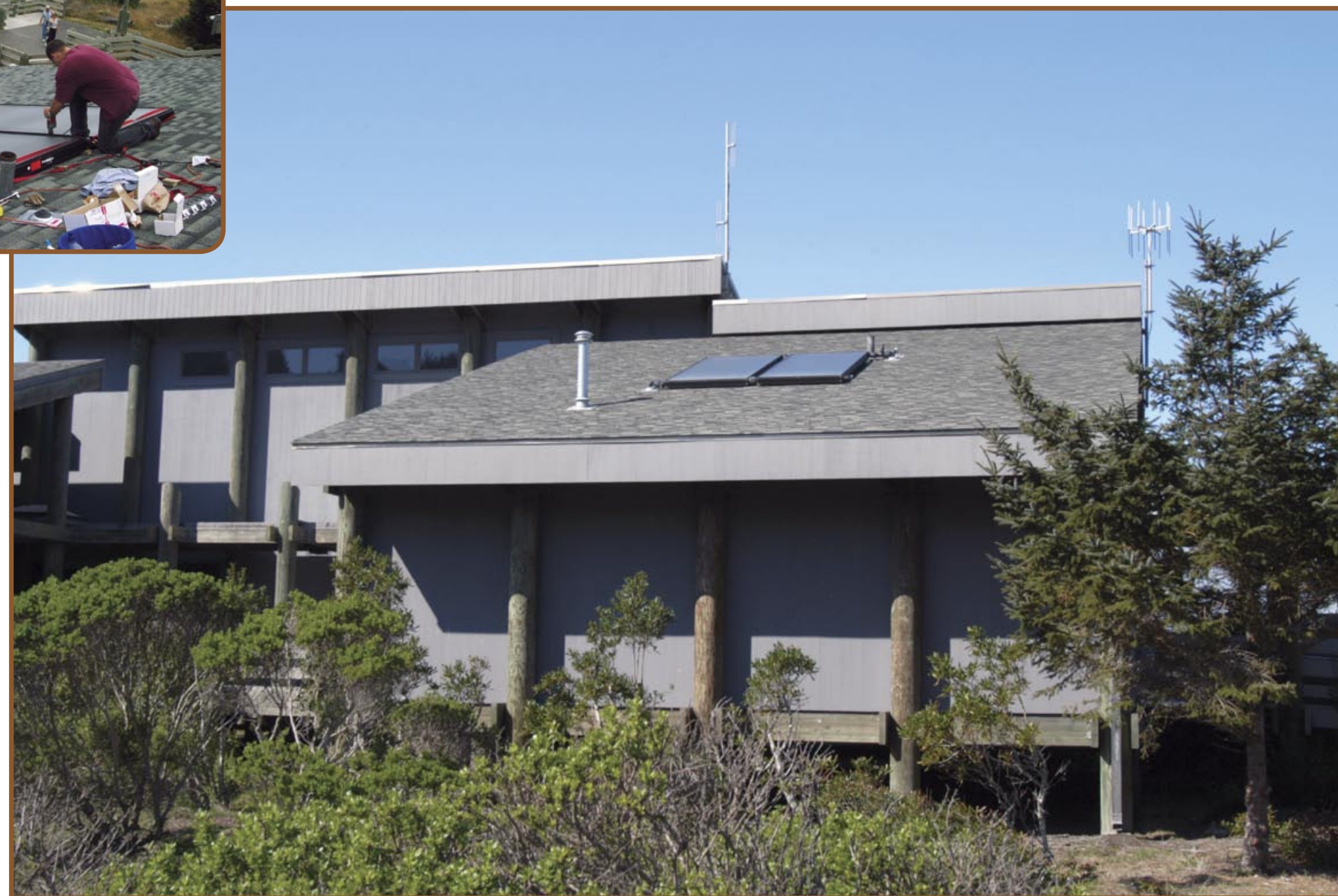
The Kuchel Visitor Center's solar hot water system was installed in 2002, providing reliable hot water for park offices and restrooms.
